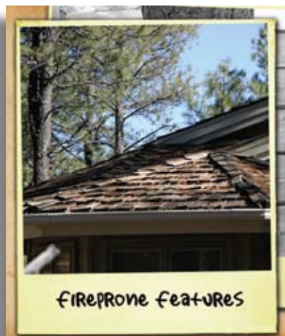
Use of flammable roofing materials
